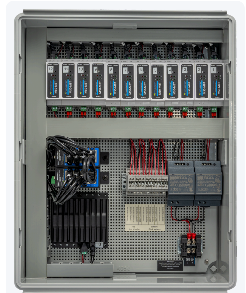
Inside the panel. Twelve IGM channels across the top, the DM processor, the built-in Ethernet switch and dual 24 VDC supplies.
